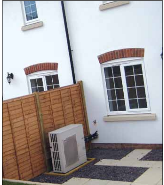
Air source heat pump
