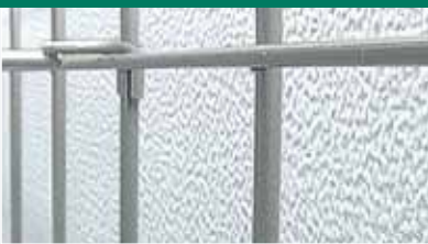
1.) Inner wall prior to the autodefrost process beginning
