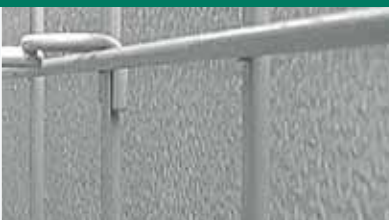
3.) Frost-free inner wall following the defrosting process
