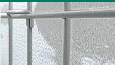
2.) Frost build-up is thawed during auto-defrost
